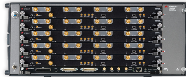
Figure 2. Five M9703B AXIe 12-bit digitizers installed in the M9505A 5-slot AXIe chassis to form a 40-channel 12-bit acquisition system.
